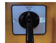
Multiple voltage selection on the panel
