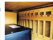
Perforated plate and rock wool within canopy
