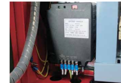
Battery Charger Enables the battery to be in constant recharging in which the generator set can be started at all time
